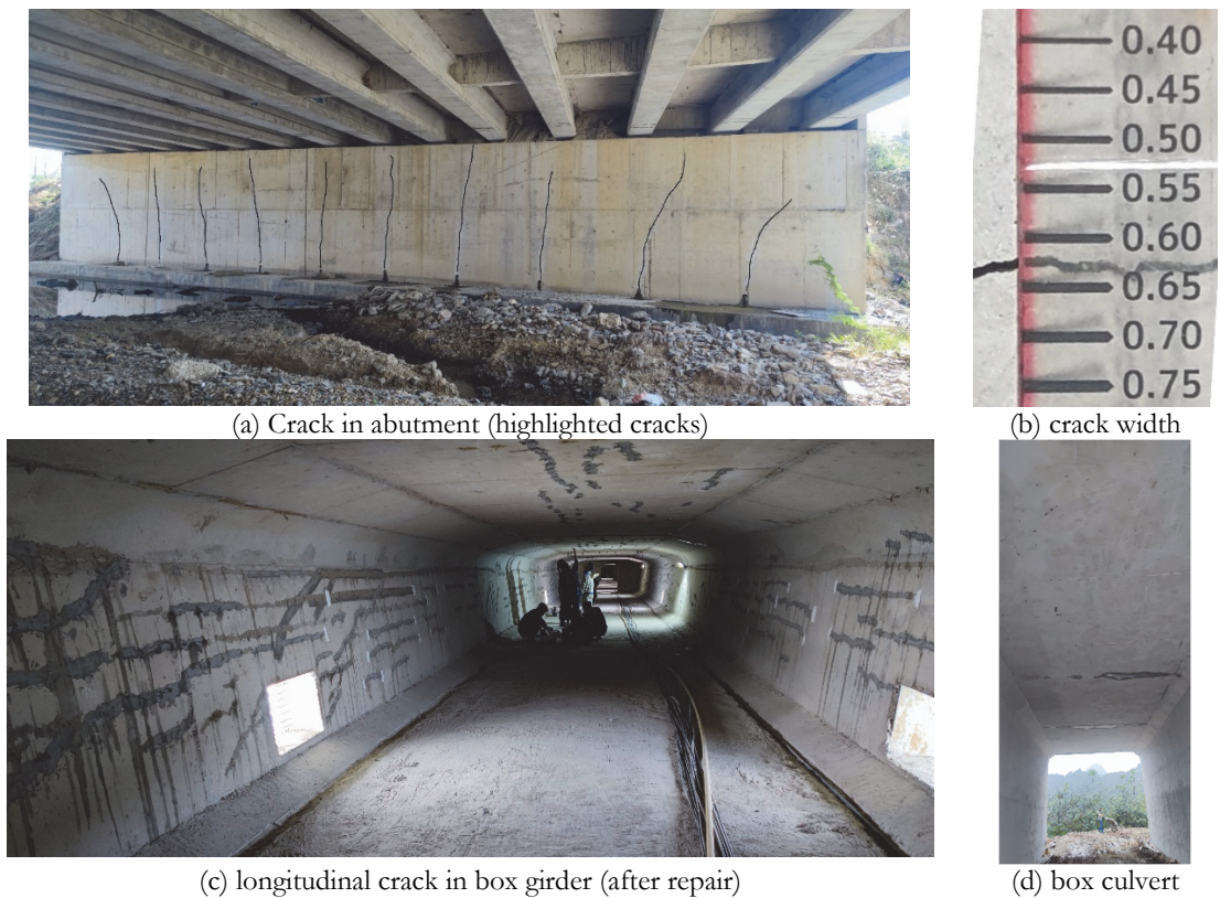
Figure 1: Typical cracks appear in bridge structure (Cracks in Fig. 1.a were highlighted).
