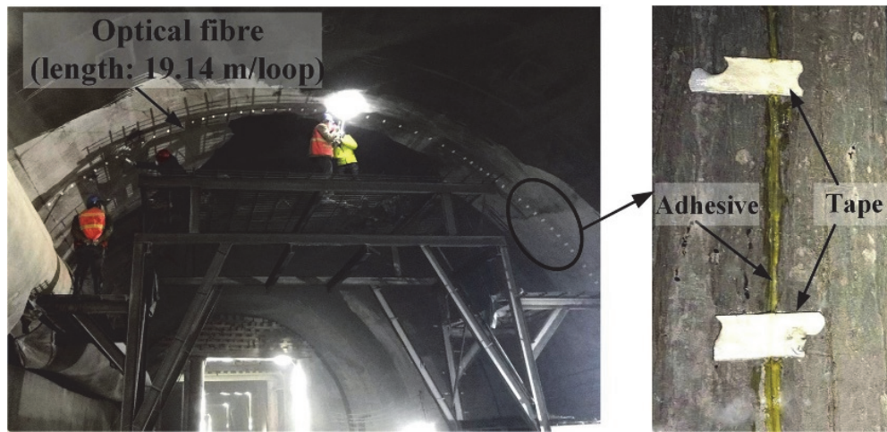
Figure 9: A view of fiber optic sensors installed in the Kaidagu tunnel lining (after Sui et al. [77], with permission from Elsevier).
